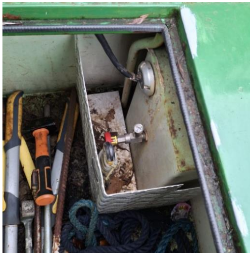
Engine bay fire suppression system manual activation plunger
