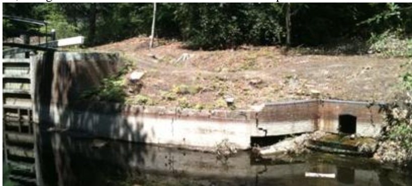
The lower wing wall of Lock 19, showing cracking and structural failure. Repairs were due to start in April this year, but are delayed yet again.
