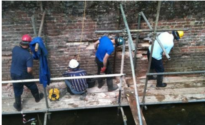
Volunteers from the Canal Society removing damaged bricks and loose pointing from the chamber of Lock 17.
