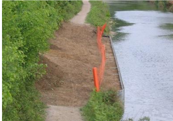
The nearly-completed 30m long permanent mooring built by Society volunteers at Runway's End, viewed from Eelmore bridge.
