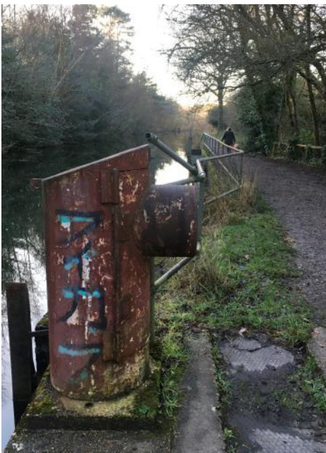
The only remaining evidence of the pumping station to Pyestock from the canal.
