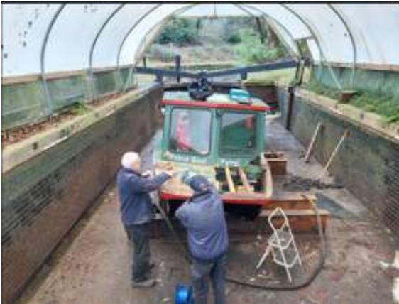
Volunteers working on the Patrol Boat with scrapers and power tools. The appropriate PPE (face masks, safety glasses & gloves) were all supplied by BCA .
