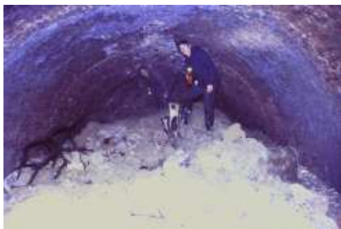
Greywell Tunnel Blockage, Tree Roots
