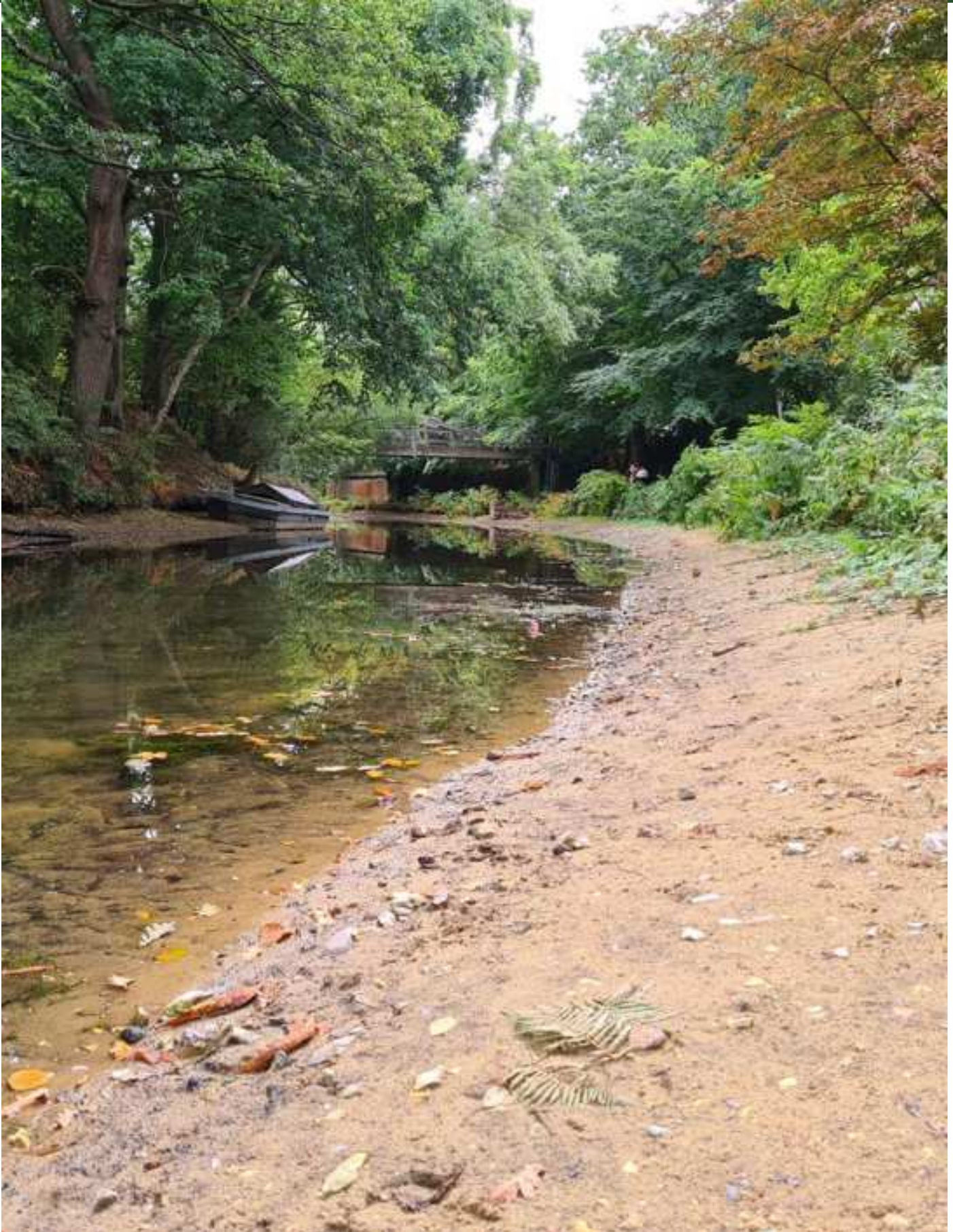
Deedman's Bridge near Mytchett Lake showing why all boating was stopped on this pound. Photo by Derek Taylor
